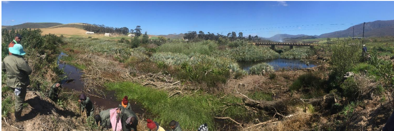
Clearing of alien invasive vegetation by Working for Water is an intervention that is aligned with EbA goals. Leveraging the success of programmes such as these can help to mainstream EbA implementation in South Africa. Pic: Alana Rebelo
